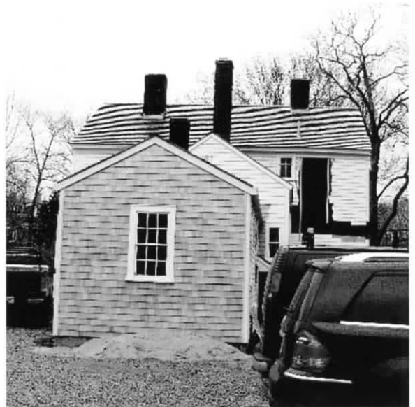
Rear view of 16 Main St. showing the ell under restoration. The ell houses a three-holer. Photo by E. Graham Ward.
