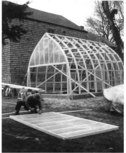
Lou Larrey works on constructing the first Outreach building, January, 1999. Photo by Paul Ferris Smith.
